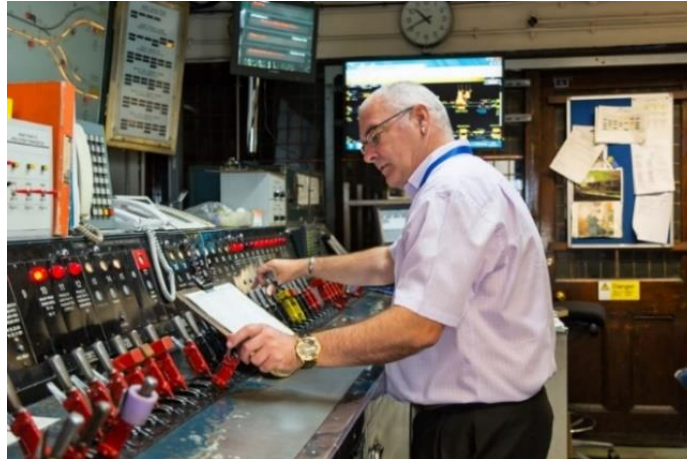
Figure 2 - Edgware Road signal cabin in operation [4]
